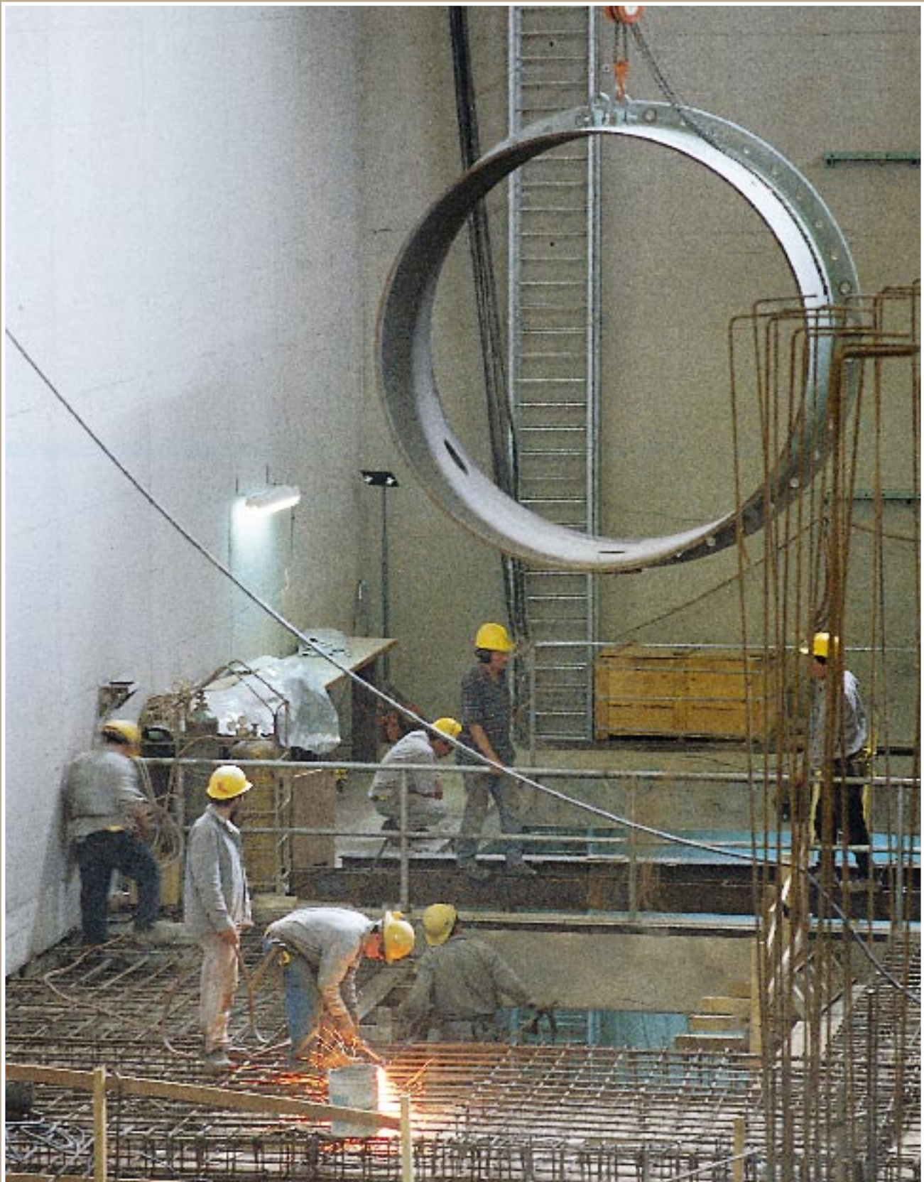
COSTA RICA—Workers install pipes in the powerhouse of the Angostura hydroelectric project in Turrialba. This project is part of the IDB's Third Power Development Program, which also includes a wind-powered project, network extensions, and an energy-efficiency commercialization project.
